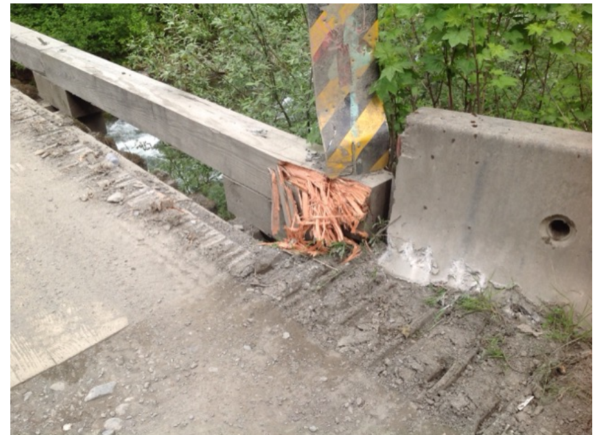
recent damage to upstream left approach rail
