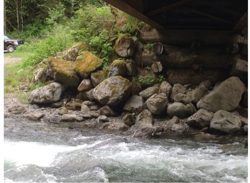
right bank downstream riprap scour
